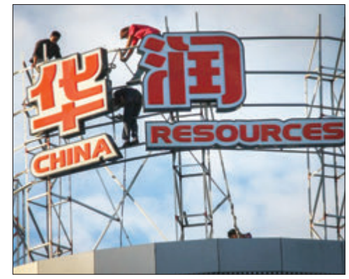
Workers install the logo of China Resources Corp in Nantong, Jiangsu province. PROVIDED TO CHINA DAILY
