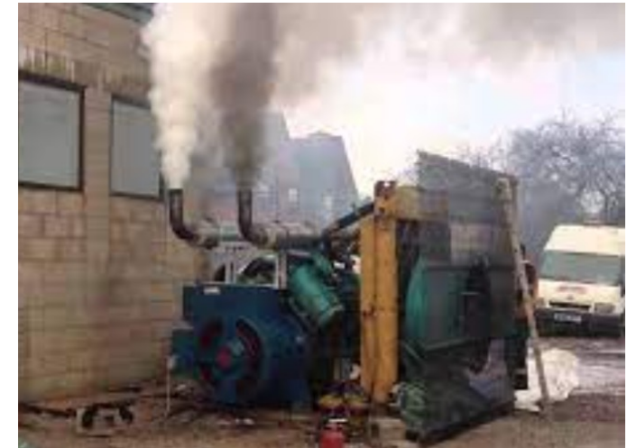
Diesel-powered emergency generators
