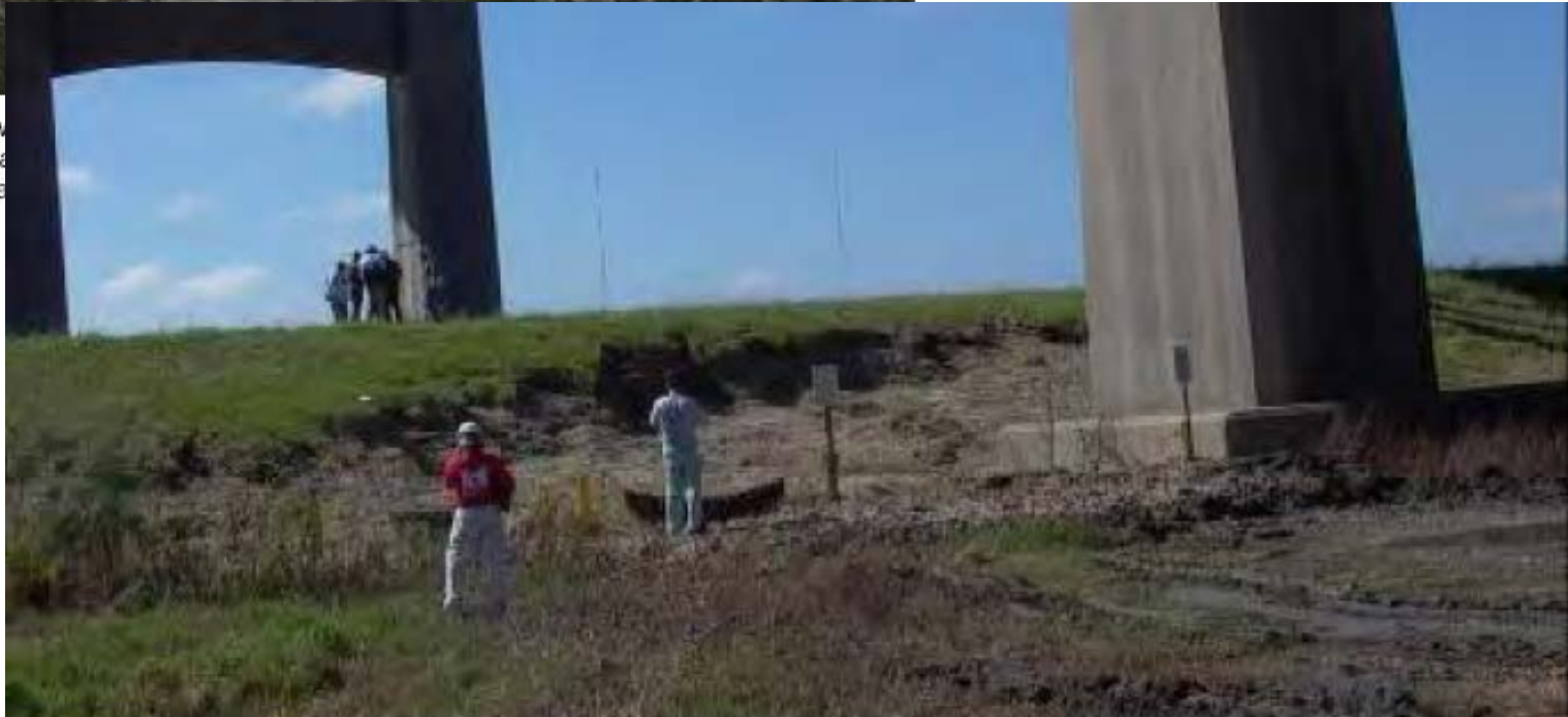
Figure 15-39. Photograph shows damage to the levee. The direction of the waves is not known with certainty, but they are thought to have come from the southwest. Waves are
